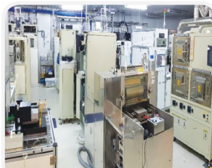
Semiconductor Display FAB (fabrication facility)
